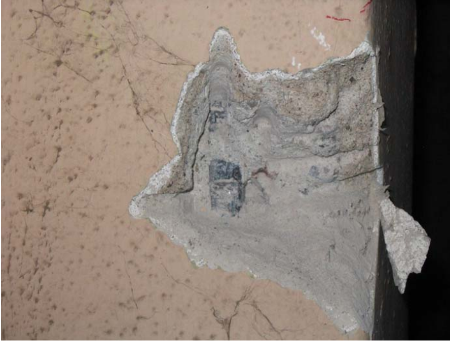
Figure 5. Exposed reinforcing bar in corner of concrete column
