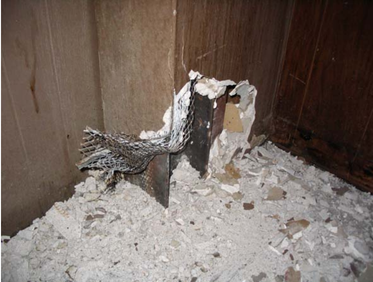
Figure 2. Plaster and lathe removed from column base to expose steel cross section for measurements.
