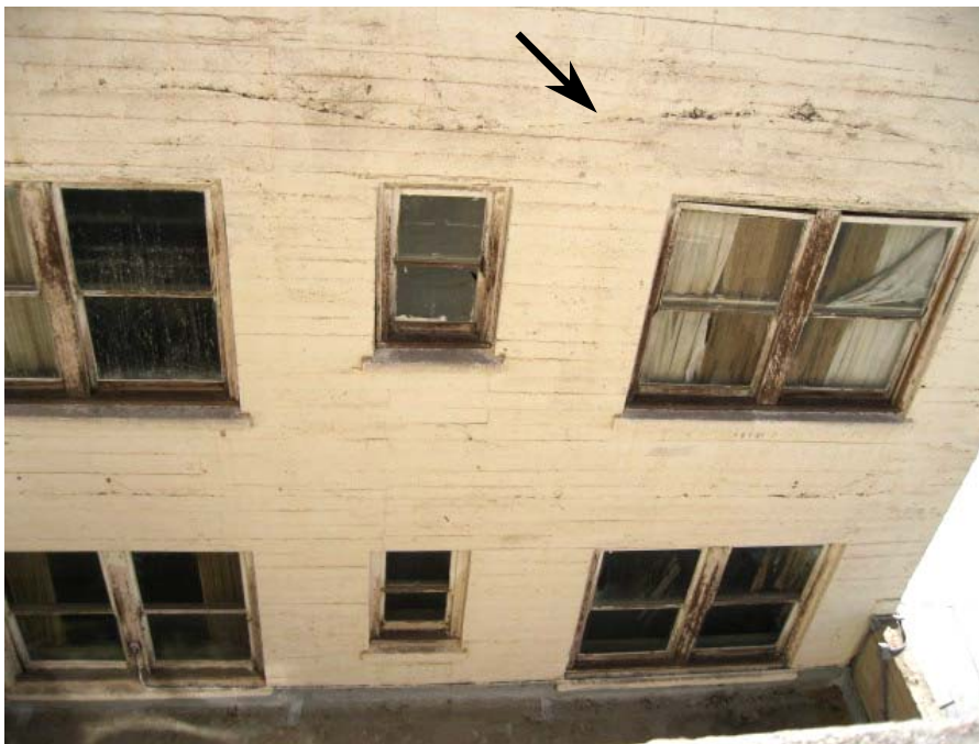
Figure 6. Typical cold joint (west elevation of west light well) as found on most elevations. The interface between successive concrete pours is not well consolidated.
