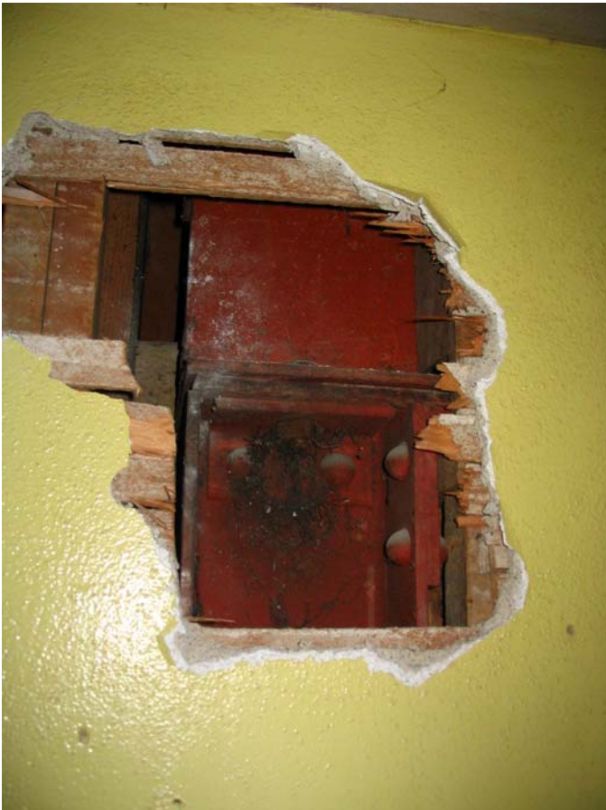
Figure 3. Top of column and end of beam visible in opening. Most connections are riveted, however bolted connections were also observed.
