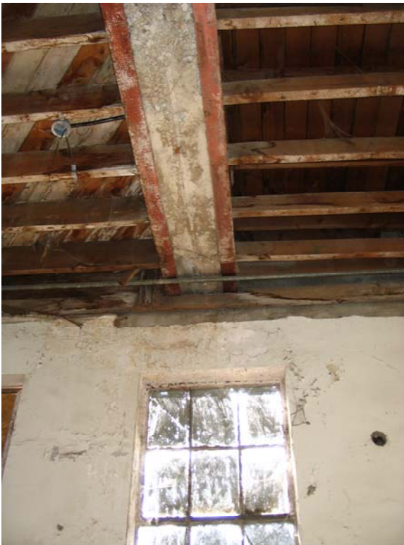
Figure 1. Concrete beam at Gridline 4 at south exterior wall. This beam supports the concrete walls on the second and third floors. Note bearing location above window head at exterior concrete wall.
